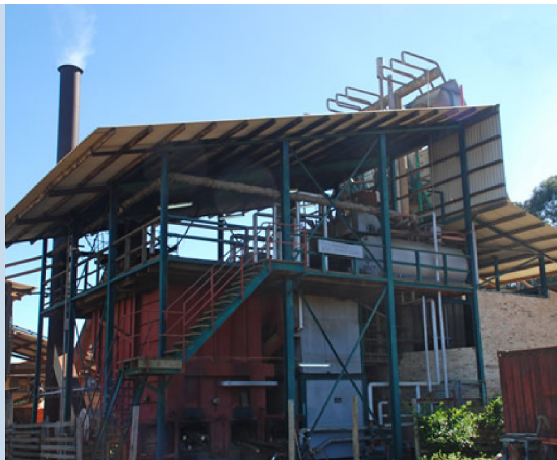
Sao Hill CHP Plant, Tanzania
